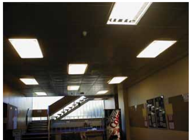
Fig.3 Ceilings appear dark with flush/recessed luminaires
